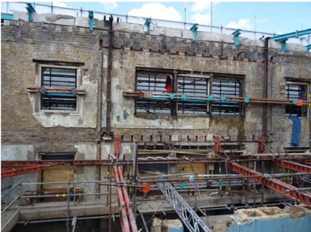
Image showing rear face with decaying brickwork, rotting timber and corroded metalwork.
