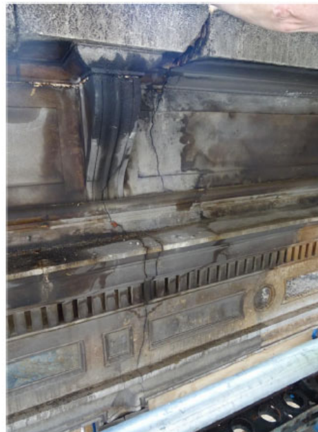
Cracking through all major stone pieces at a structural node in the façade.
